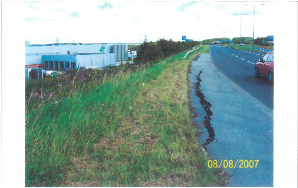
▲ Photograph 1 – The cracked footway looking west (August 2007).
