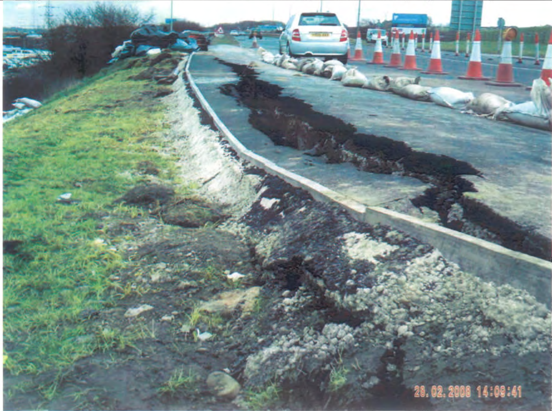
▲ Photograph 2 – The cracked footway looking west (February 2008)
